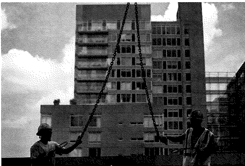
Contractors load steel rebar at the construction site of a residential building in New York, on Aug. 11, 2016.
